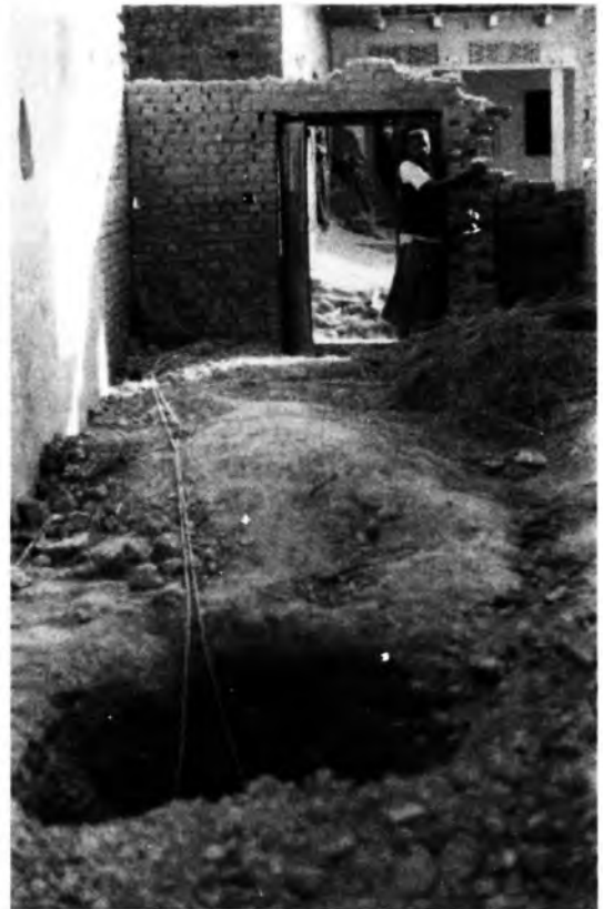
Photo-3 Outer rim of collapse land in the premises of Shri Prabhunath Singh, Karanda Village, Ghazipur District, U.P.
